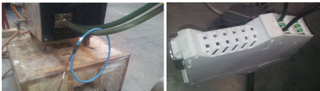
(a) (b) Fig.14 Installation of Rogowski coil and integrator for induction heating
